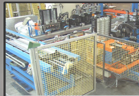
GENERAL VIEW OF SEAMING BENCH
